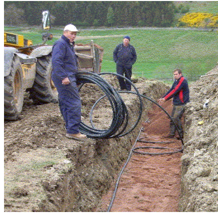
The straight pipe is the outward flow pipe, the curled pipe is the return flow pipe
